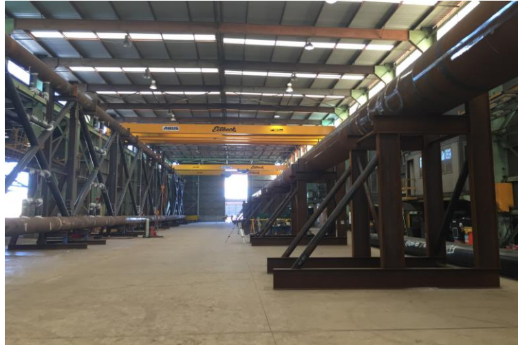
Figure 3: Bottom and top chords/bays lifted into their correct horizontal and vertical alignments. These alignments were positioned by survey. Inter-connecting bays at this stage were only tack/pre welded together as a part of the trial fit.
