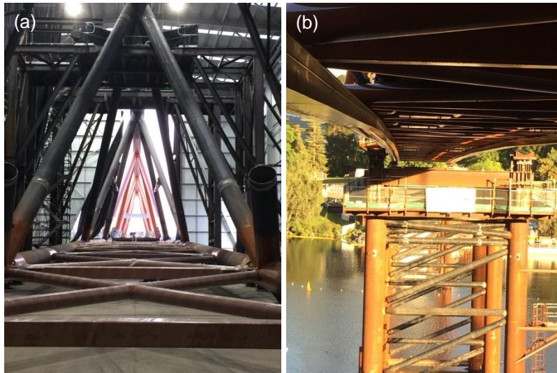
Figure 17: (a) View of triangular shaped truss being re-assembled in sections, and (b) nodes being supported during launch vary due to the vertical alignment.
