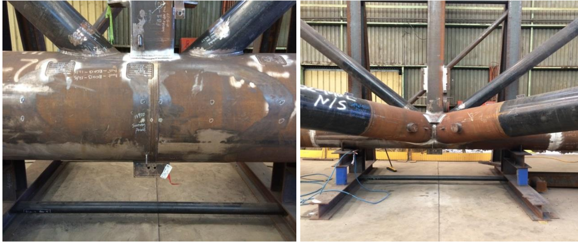
Figure 13: Adding pipes to the truss caused punch marks to be destroyed.
