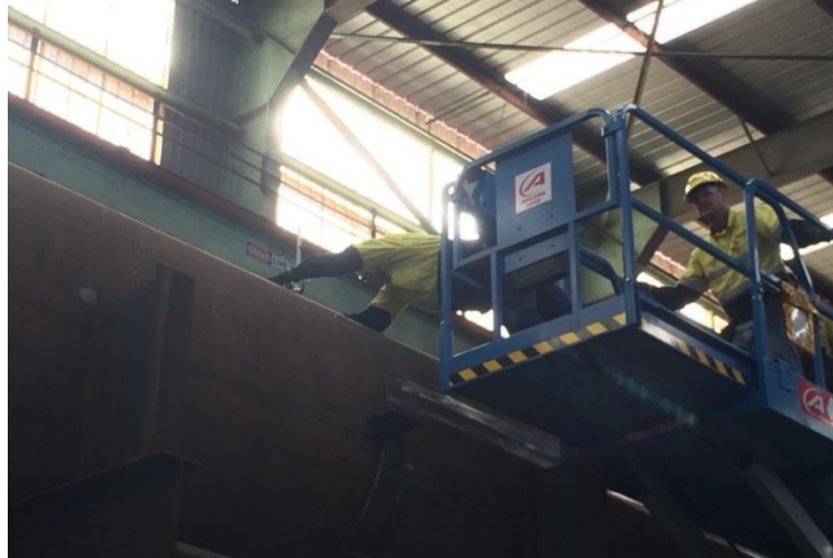
Figure 11: Taking a measurement on top of a pipe suspended 4 m or higher above the ground.
