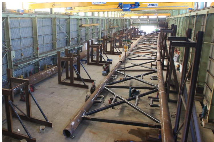
Figure 2: Manufacturing of top and bottom chords/bays. These we surveyed to ensure correct lengths and grades.
