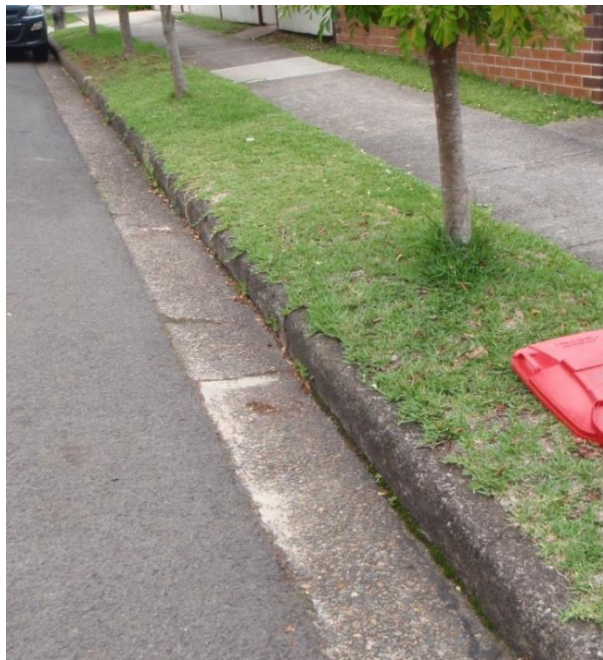
Figure 16: Section of very old concrete kerb in Cambridge Street, which was monumented (to the kerb line between stone alignment posts) in DP370103 (1950) and has been used ever since for definition.
