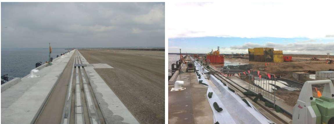
Figure 5: Dramatic change in site conditions from Phase One to Phase Two of construction.
