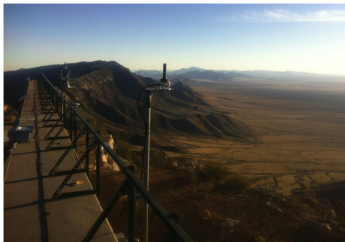
Figure 3: One LocataLite installed on a mountaintop at White Sands Missile Range.
