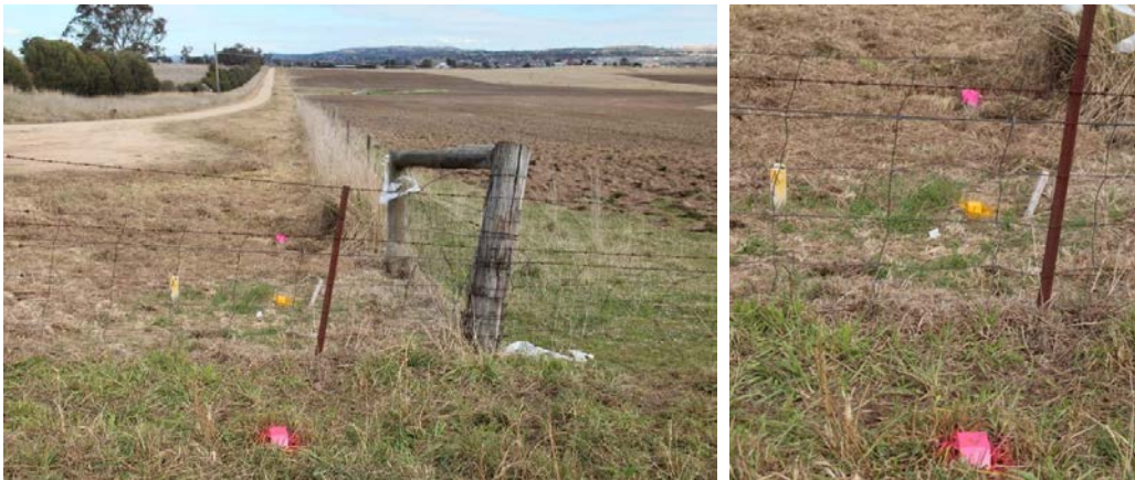
Figure 9: Offset pegs (pink 75 x 75 mm) and pillar peg (yellow 75 x 75 mm) plus Telstra peg (yellow 32 x 75 mm) at Pillar 7. All cable locations were potholed before boring.
