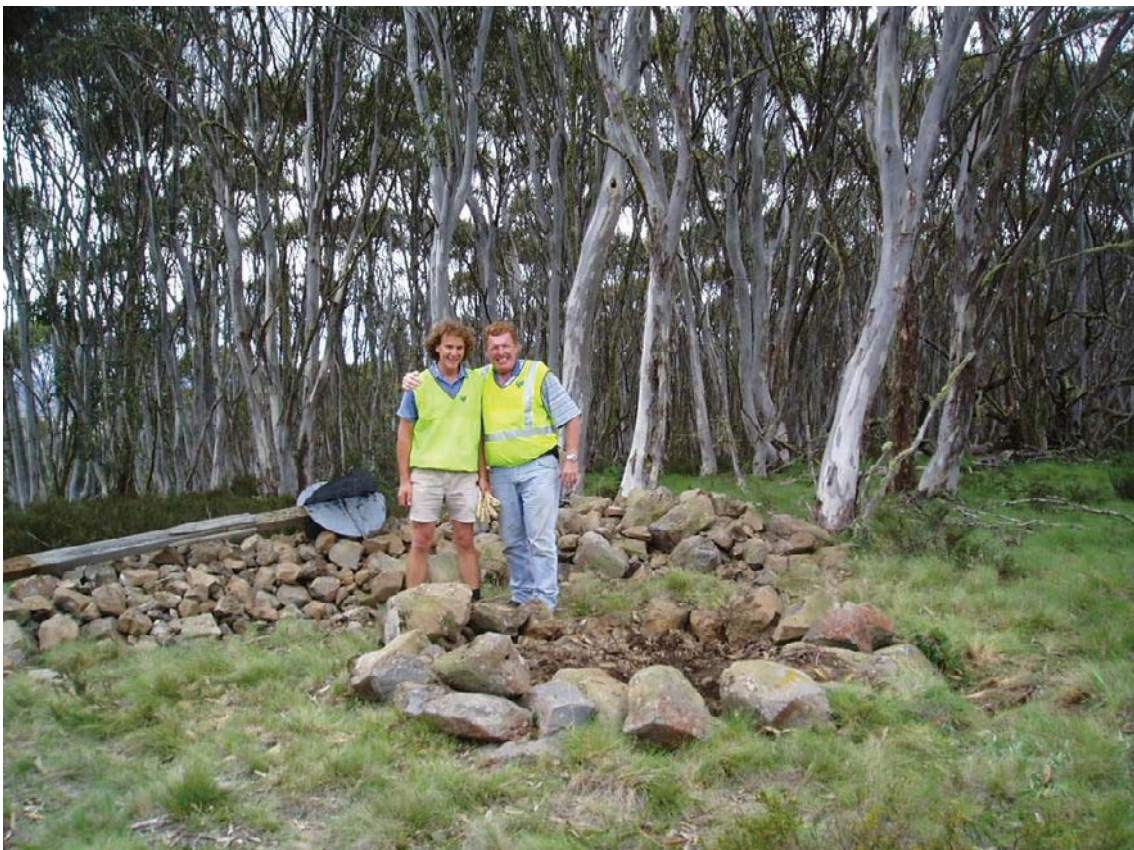
Photo 5: And ultimately, here's what the "Demolition Team" (Alex Gillies and Pete Radley) had to do for us to be able to use it!
